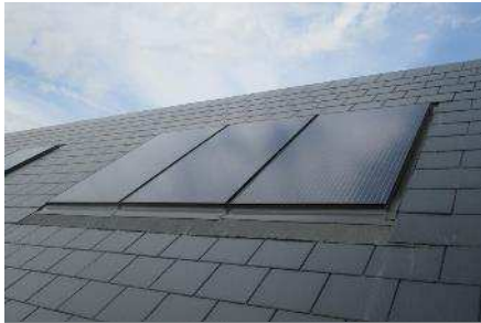
Photovoltaic (PV) panels
