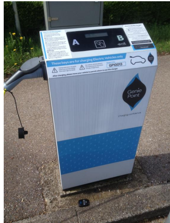
Existing 2 x Chargepoint Genie 7kW unit as installed at South Winchester Park and Ride
